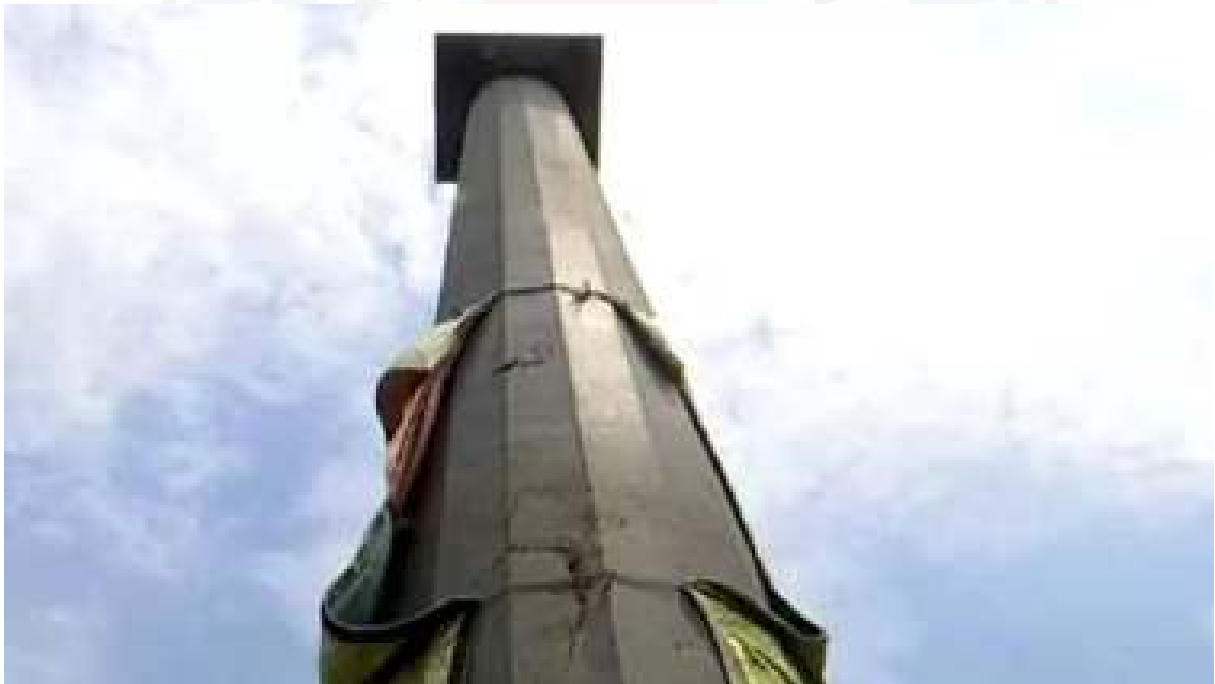
Cracks being seen in the Aruna Stambha present in front of the Singhadwara on August 28, 2022.
