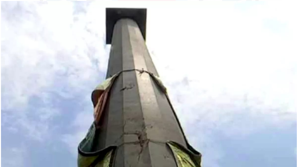
Cracks being seen in the Aruna Stambha present in front of the Singhadwara on August 28, 2022.
